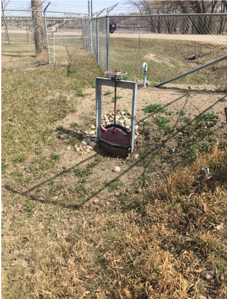
Photo 1 Example of manually operated shut-off as a control gate from SaskPower's Queen Elizabeth Power Station located in Saskatoon, SK
